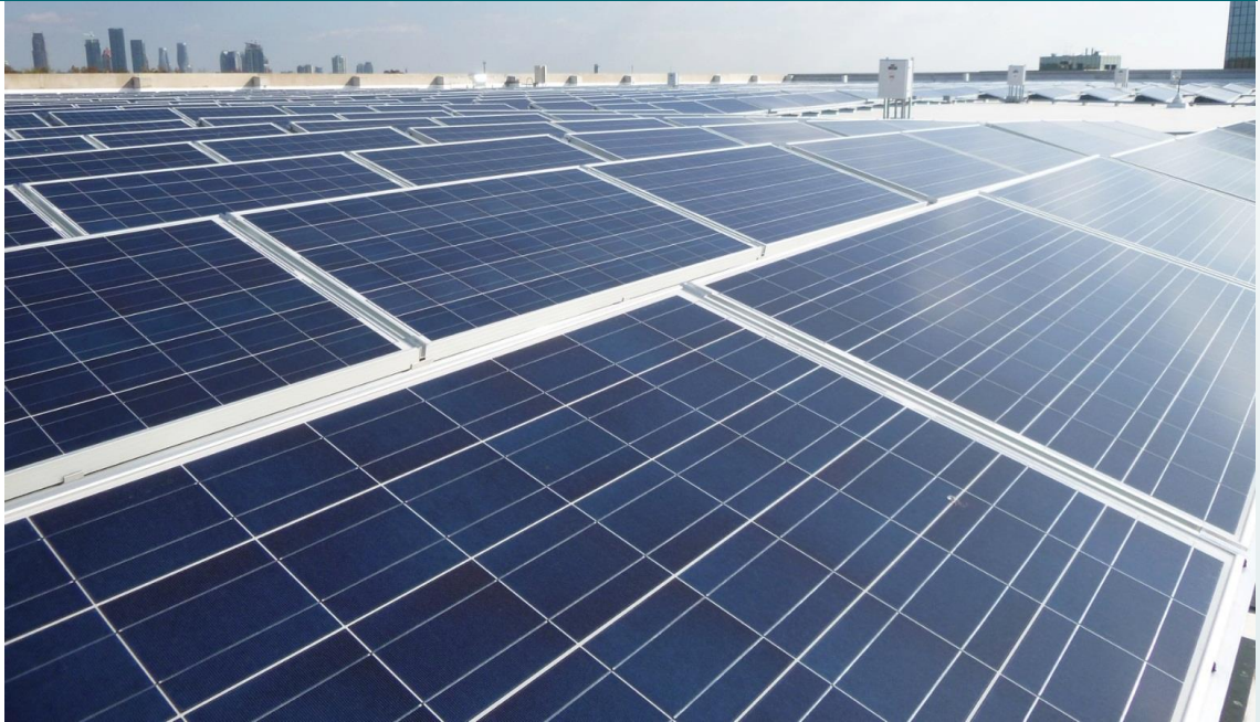
Metrolinx – Erindale Station | 300 kWp
